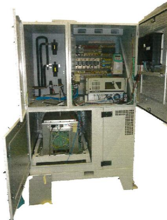
MOD-8000 (doors open, air conditioning door closed)
